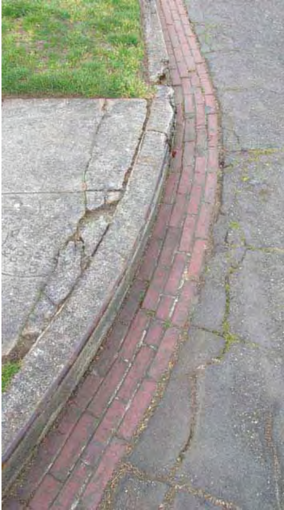
Example of brick gutter, N. Cedar Street north of N. 15 th St.
